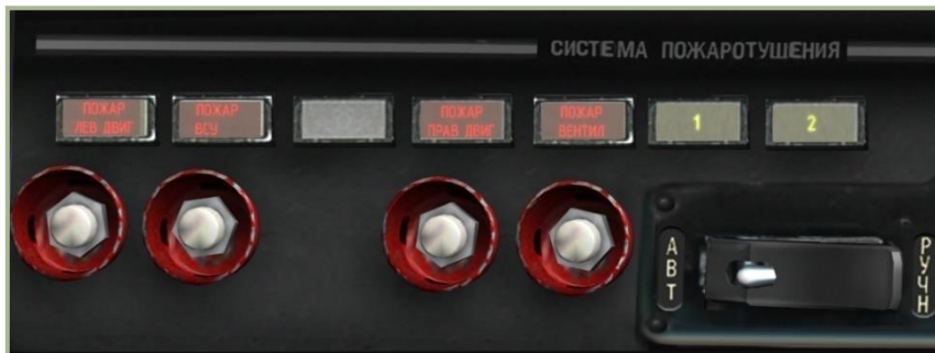
10-19: Fire extinguishing system control panel
