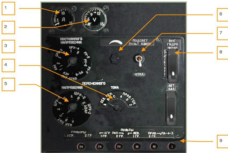
6-71: Electrical System Control panel
