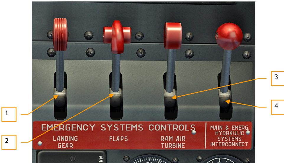
Figure 53: Emergency hydraulic system valves
